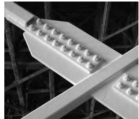
Cross bracing protected with intumescent coating
